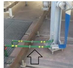
Fig. 1. Iron solid iron conductor, which used for earthing in power station [7]
